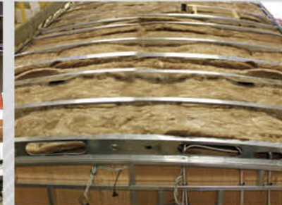
Aluminum truss roof system
