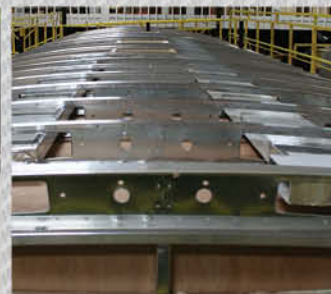
Walkable steel truss roof system
